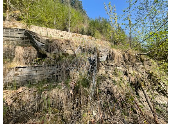
Failed grs wall
